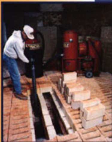
Brick manufacturer uses INVINCIBLE unit for conveying heavy abrasive sands. Applications include cleaning out kilns (shown above), central housekeeping, spill pick-up and product reclaim.
