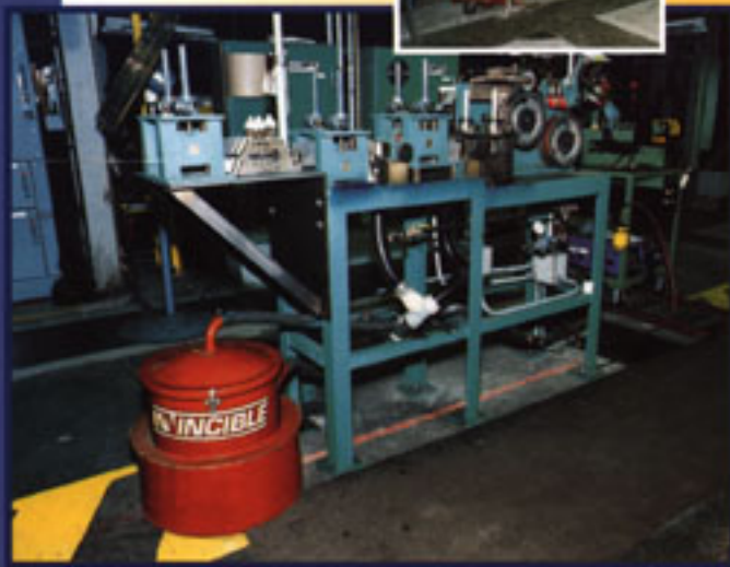
Saving shavings. A manufacturer of stainless steel products uses one system to solve two problems. Shown above is one of three stainless steel strip deburring processes all powered by a single model 4594. This system is designed to source capture and reclaim valuable shavings and provide a safer work environment.
